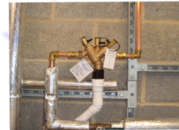
RPZ Valve installation & servicing
